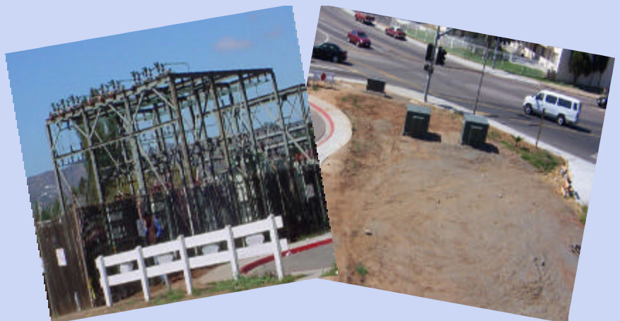
Before and After: An old energy substation gives way to clearer view for residents of Lakeside.
